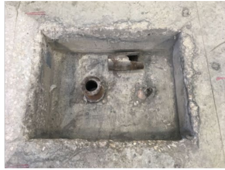
(b) Broken couple in first base
