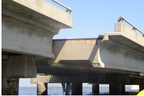
(a) Lateral movement of I-10 twin bridge, USA
